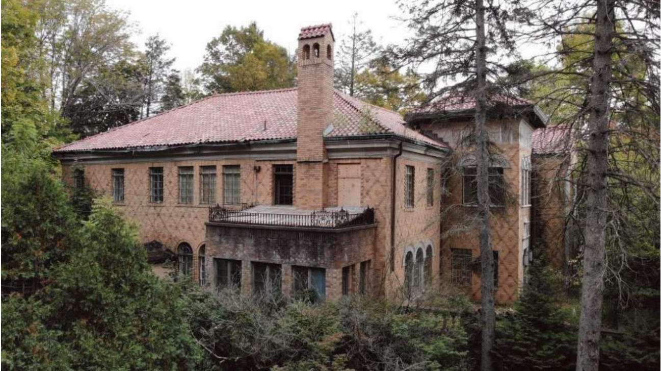
Drone Photograph - Temporary Roof over West Porch and Collapsing Gutter System and Incomplete Downspout System
