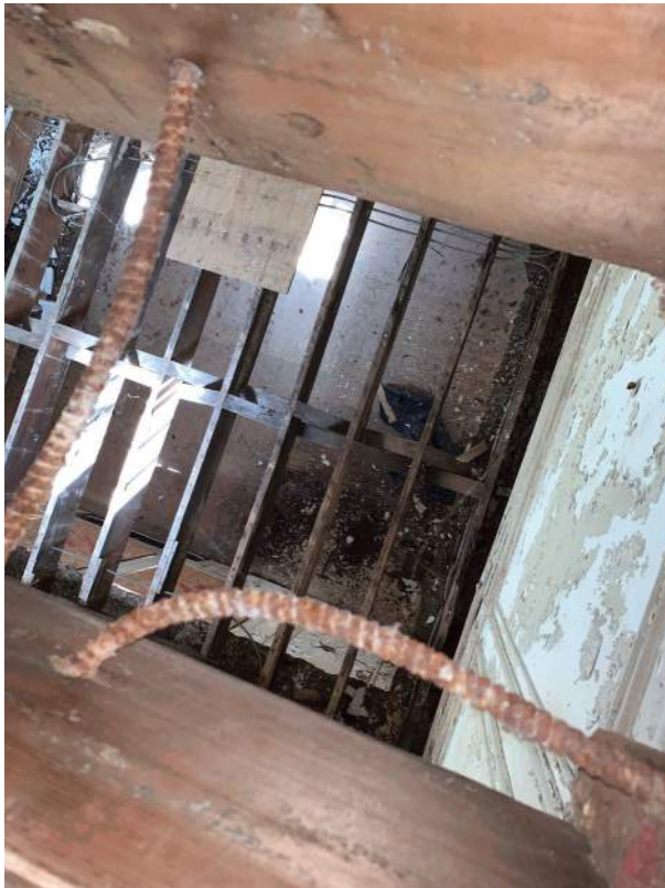
View to First Floor Level and Damage at Roof and Exterior Wall Intersection
