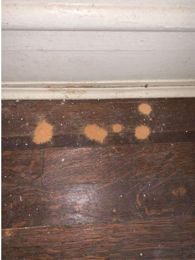
A Location in the East Wing of the Second Floor Level, Where the Flooring and Walls Seem to be Original and Intact, Shows Signs of Powder Post Beetle Activity
