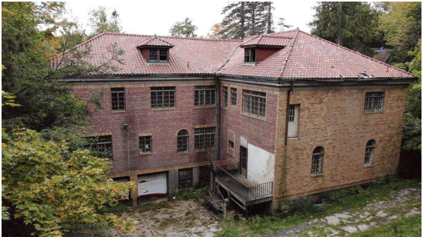
Drone Photograph - Main Building North, Roof Mostly Intact and Collapsing Gutter System and Incomplete Downspout System
