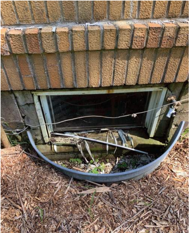
Example of Altered Basement Window Opening and Deteriorated Replacement Window
