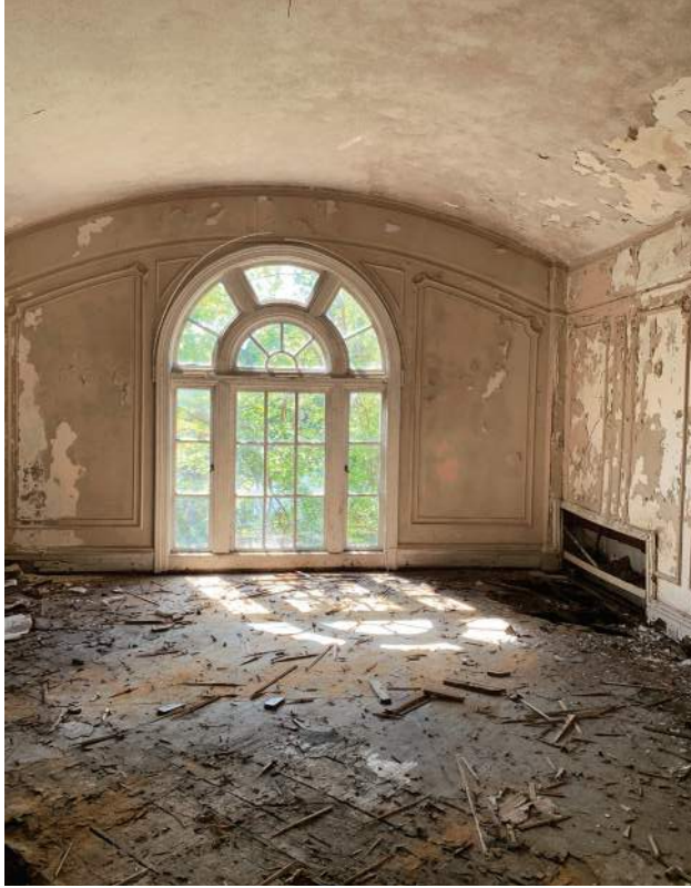
Bedroom No. 1 Damaged Floor Around Inwall Radiator Beneath a Roof Gable and Exterior Wall Intersection
