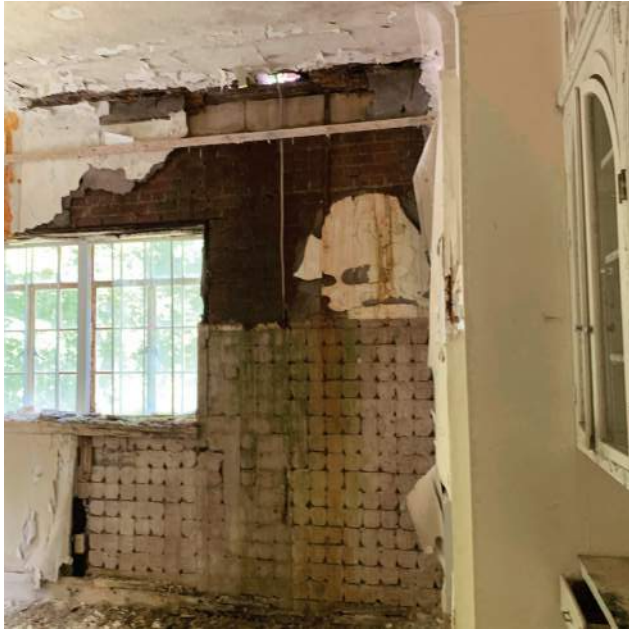
Second Floor Level North Wall of Kitchen Showing Missing Tiles and Roof Edge and Ensuing Damage
