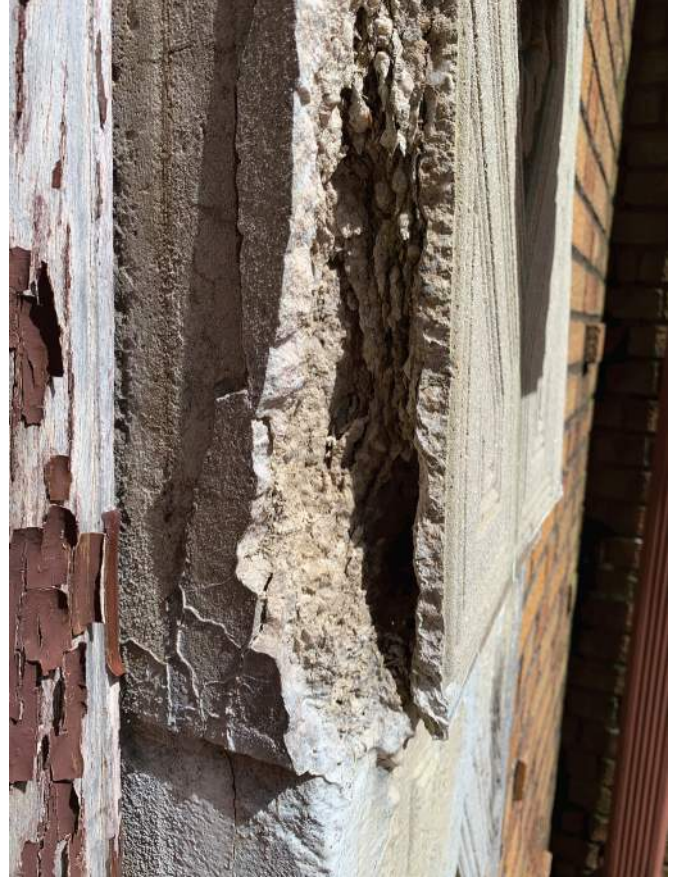
Deteriorating Cast Stone Building Element at Door with Signs of Past Repair
