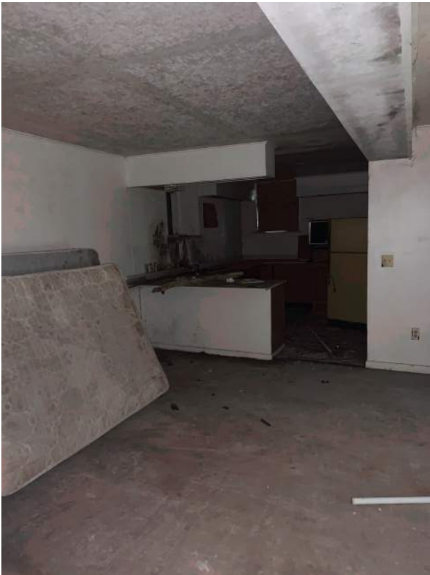
Apartment Kitchen with Window Boarded over
