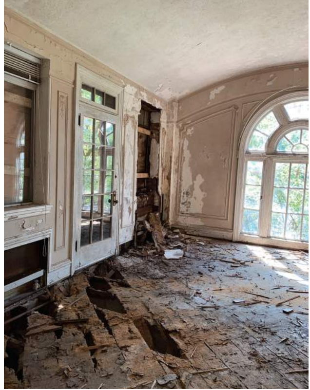
Bedroom No. 1 Damaged Floor Along Exterior Common Wall with Southeast Sunporch
