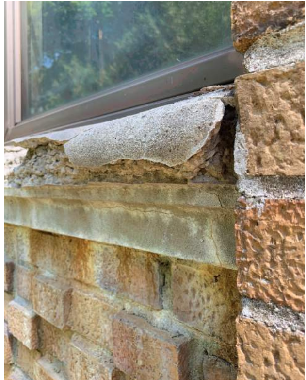
Deteriorating Cast Stone Building Element at Sunporch Sill
