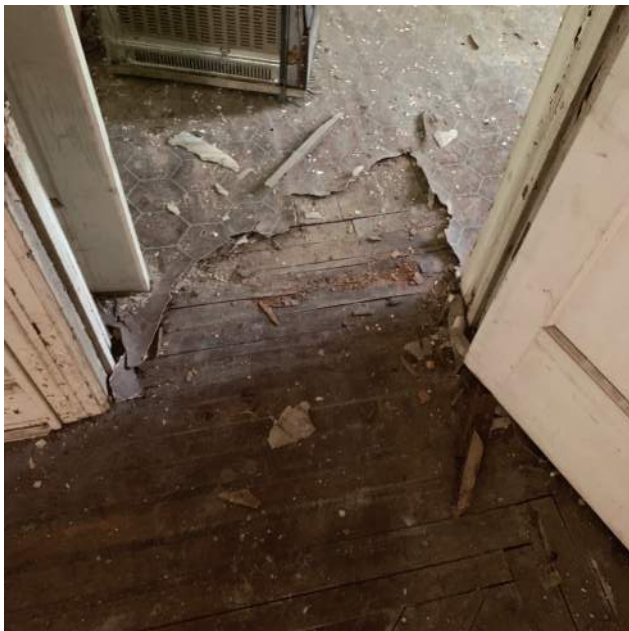
Evidence of Sheet Flooring on Top of Wood Trapping Moisture and Magnifying the Damage
