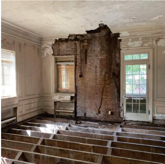
Living Room with Extensive Wall and Floor Damage Around Chimney and West Sunporch
