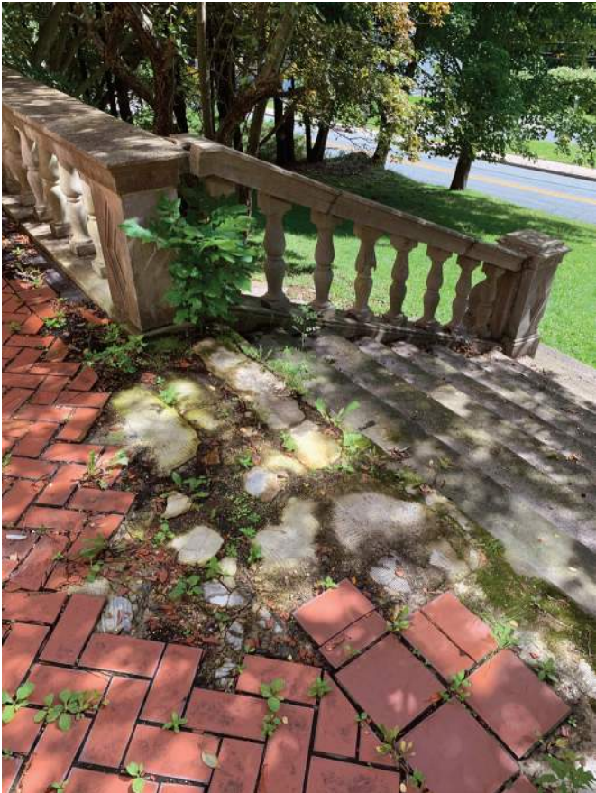
Concrete Stair up to Terrace and Main (Front) Building Entrance off of Chestnut Street
