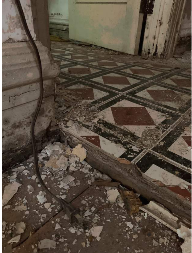
Odd Floor Level Change From Vestibule to West Living Unit
