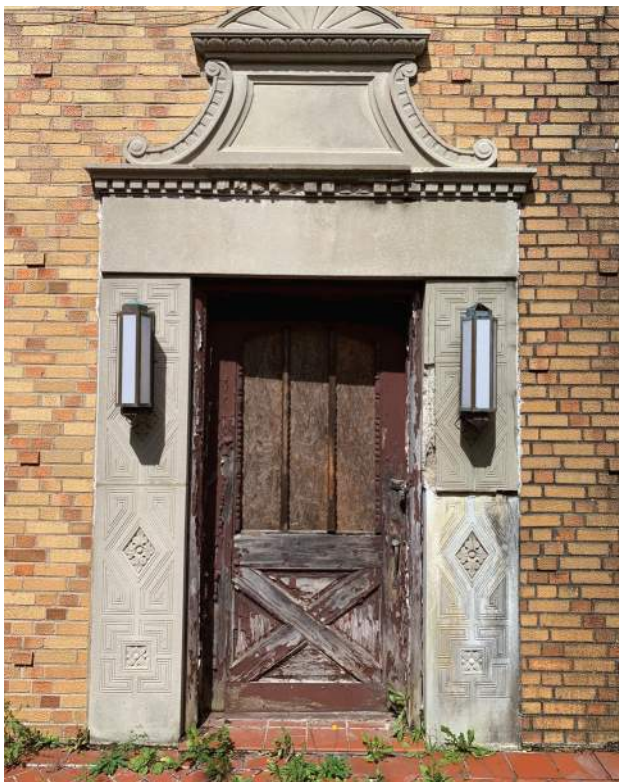
Main Entrance - Example of Cast Stone Repair and Cast Stone Replacement
