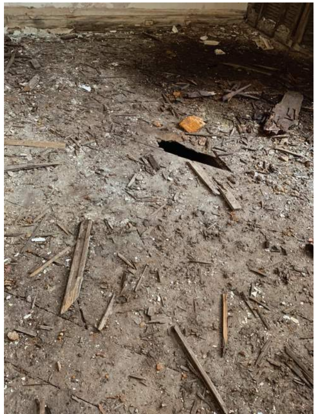
Water Damaged Wood Flooring
