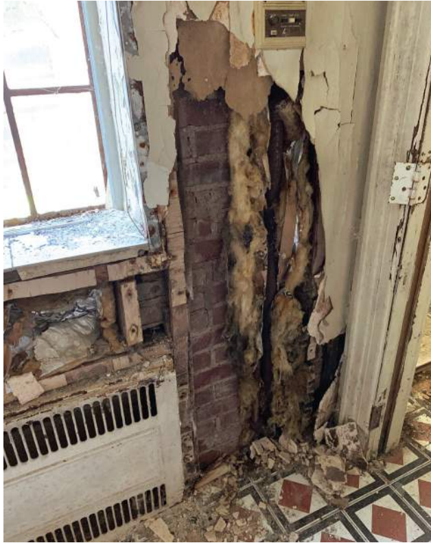
Water Damage in West Living Unit Kitchen
