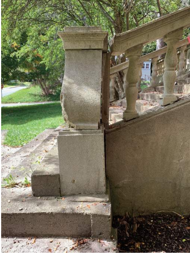
Deteriorating Cast Stone Terrace Stair Site Elements
