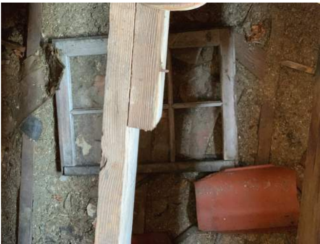
Rubble and Window Components
