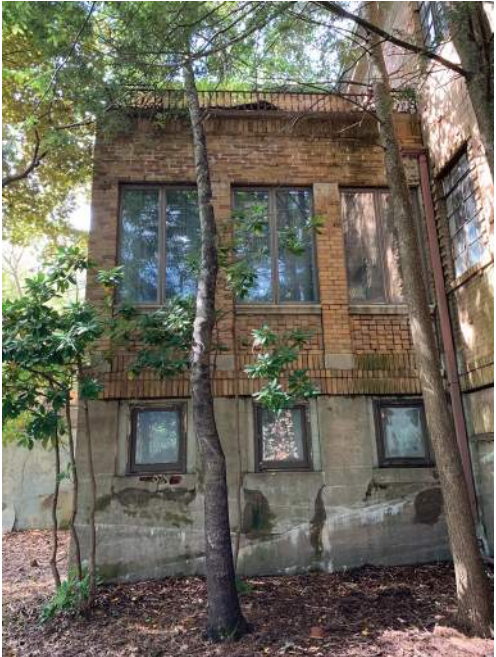
Southeast sunporch with temporary roof above – refer to first floor interior images, first floor windows are a modern enclosure of the porches typical
