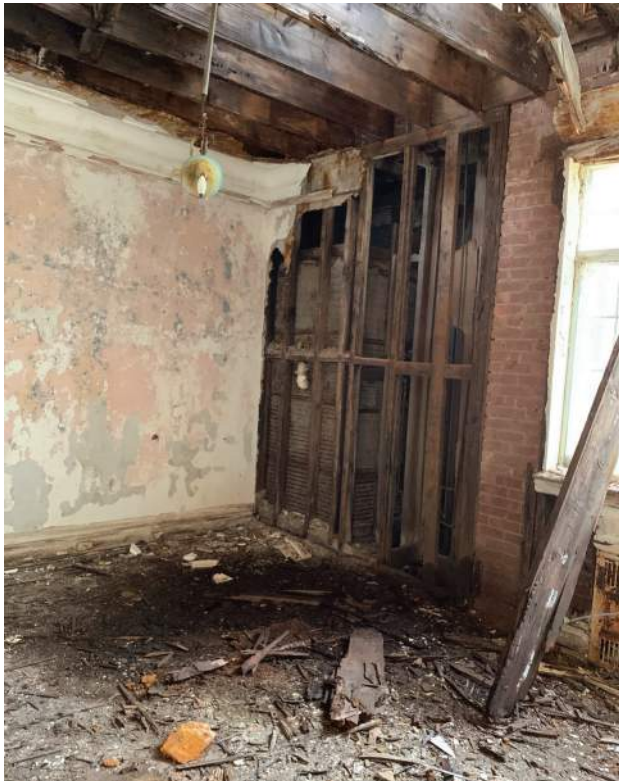
Bedroom with Water Damaged Floor and Collapsing Ceiling Joist Structure Above
