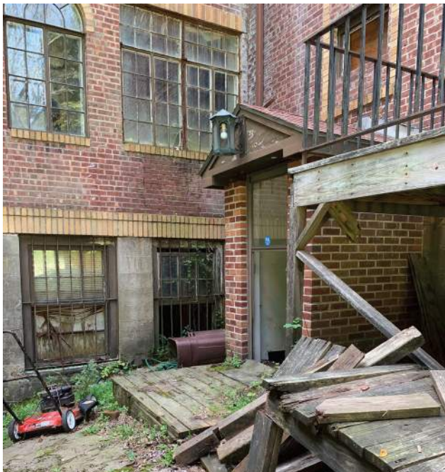
Copper Rear Light Fixture at Entrance Not Shown on Plans
