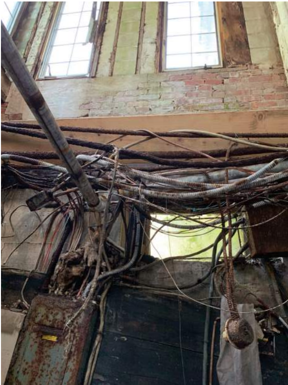
Main Electrical Service Distribution
