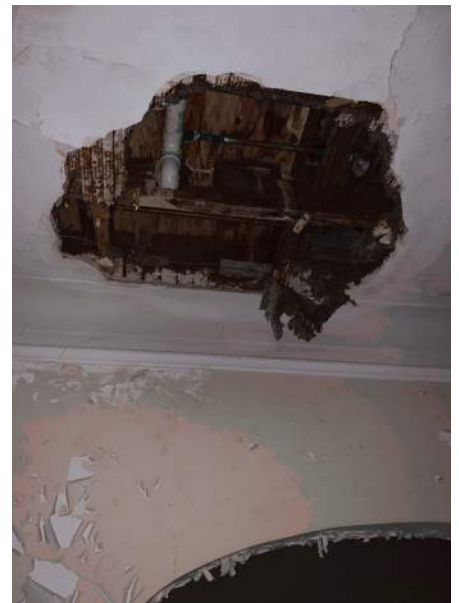
First Level Ceiling Evidence that Pipe Leaks Have Caused Damage
