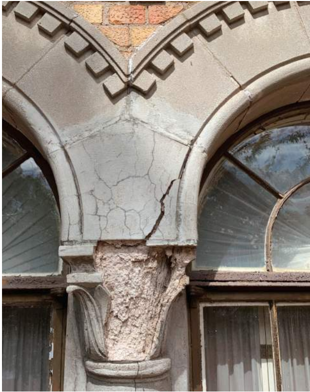
Deteriorating Cast Stone Building Element - Showing Signs of Repair at Window Hood Pilaster
