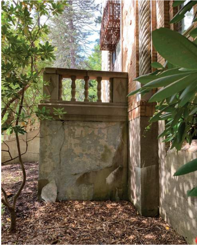
Area of the Terrace in need of Repair
