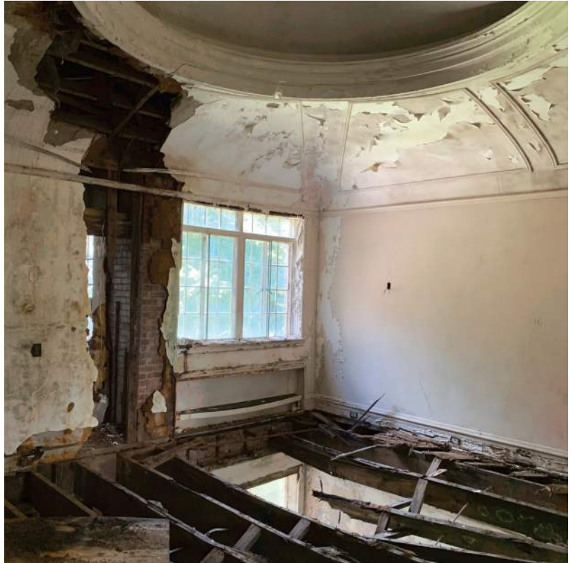
Domed Reception Room Ceiling and Wall Damage Beneath Roof Valley Flashing
