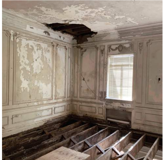
Living Room Damaged Floor Beneath a Roof Exterior Wall Intersection
