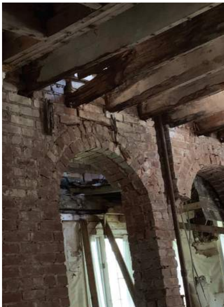
First Floor Level Living Room Ceiling Condition at Southeast Sunporch
