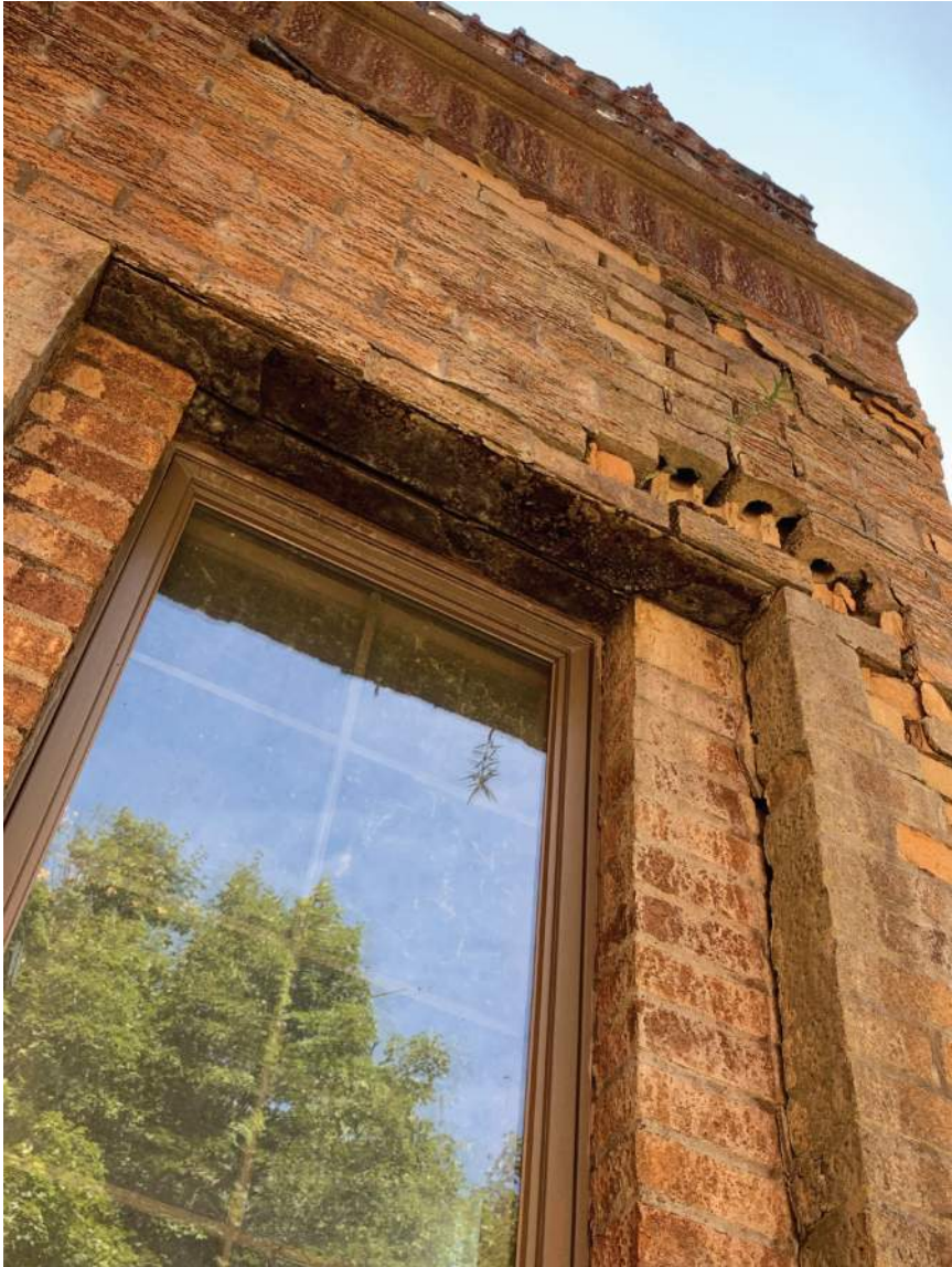
Brick Repair Required at West Sunporch Typical
