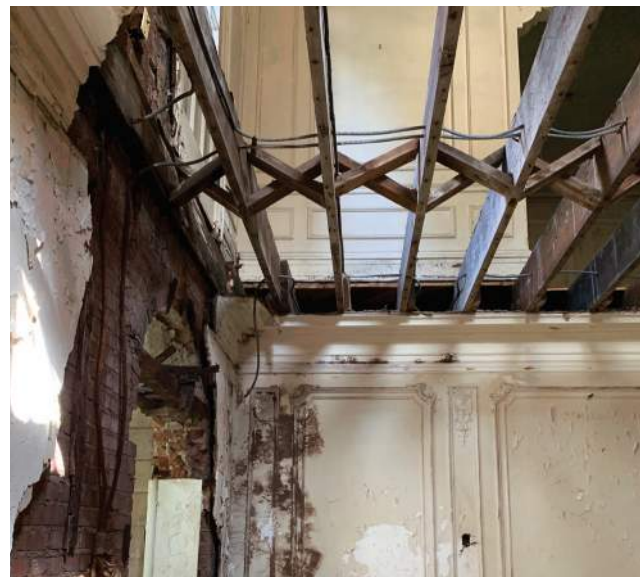
Roof Drainage Damage and View to Second Floor Level Living Area
