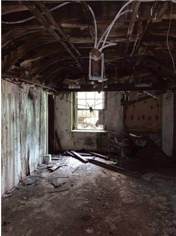
Laundry Room Showing Extensive Water Damage
