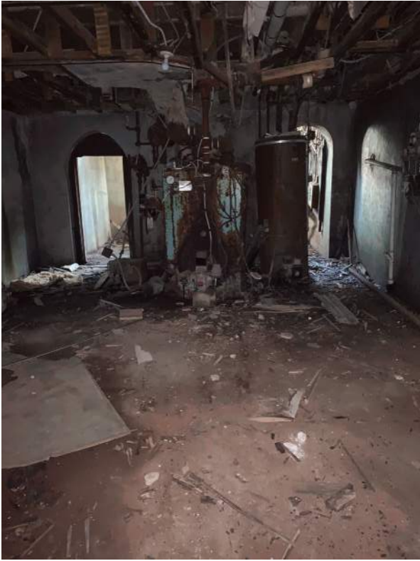
Central Boiler and Water Heater
