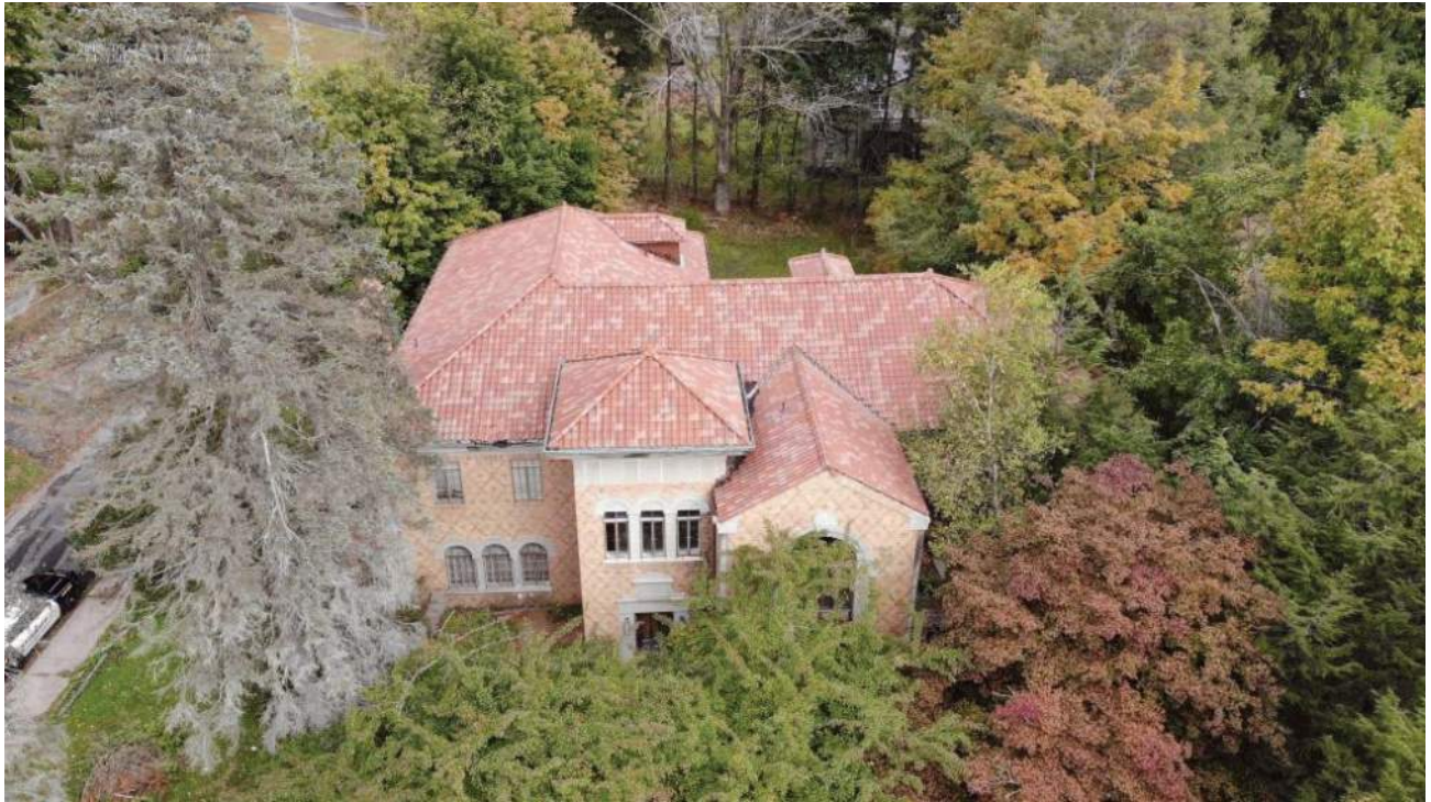
Drone Photograph - Main Building Roof Mostly Intact
