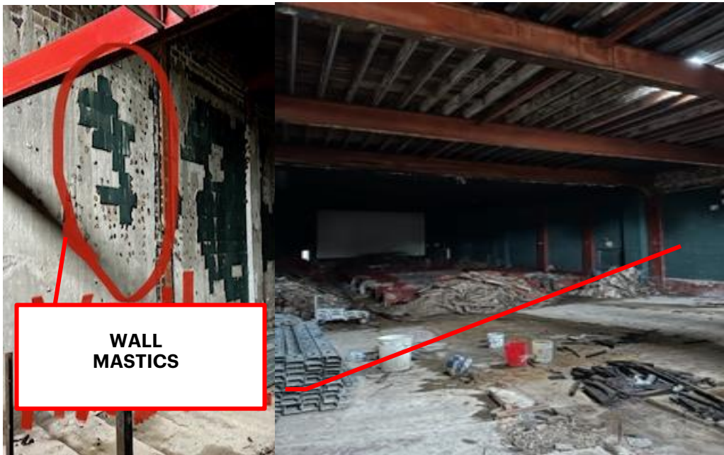
THEATRE, WALL MASTIC SIDE WALLS
