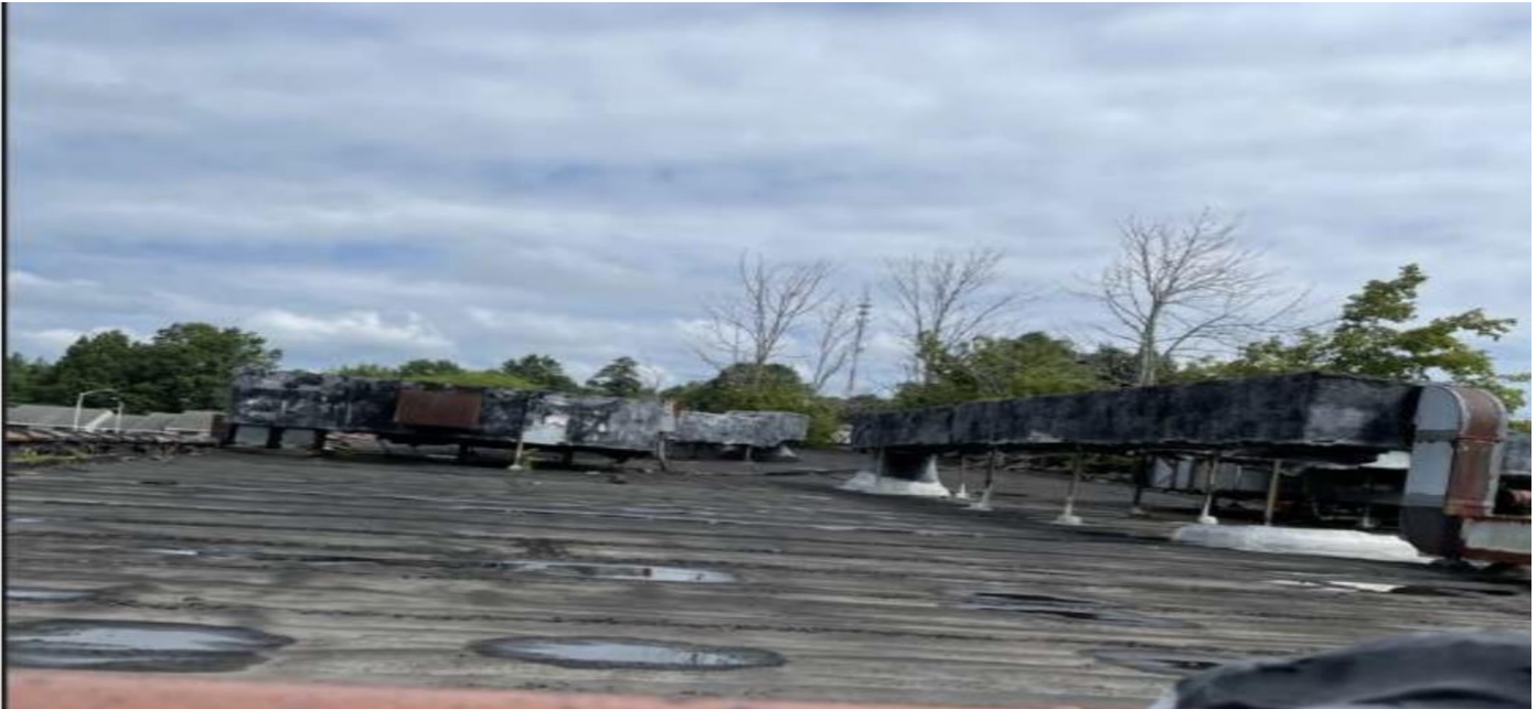
MAIN ROOF, POOR CONDITION; ASSUME ALL ROOF/MASTICS TO BE ACM
