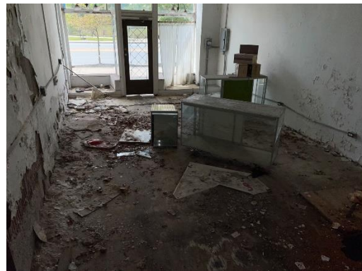
Photograph # 8 Water damaged floor and walls in Vacant Storefront #1.
