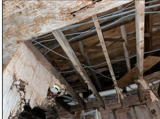
Photograph # 6 Water damaged collapsed ceiling in lobby. Roof deck by roof drain saturated.
