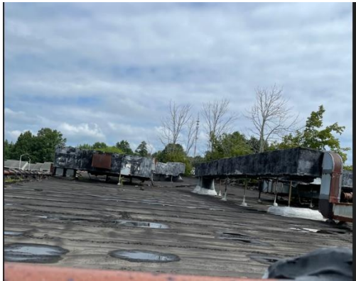
Photograph # 15 North looking view of upper roof. Pooling visible on damaged roof membrane.
