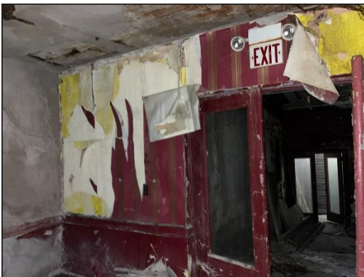
Photograph # 7 Water damaged walls and ceiling in lobby.
