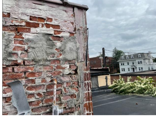
Photograph # 14 Deteriorated masonry at exterior wall.
